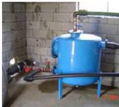
Figure 4: A treated wastewater filtration unit consisting of sand filters (in blue) and a disc filter (in black) (source: MREA, 2006).
